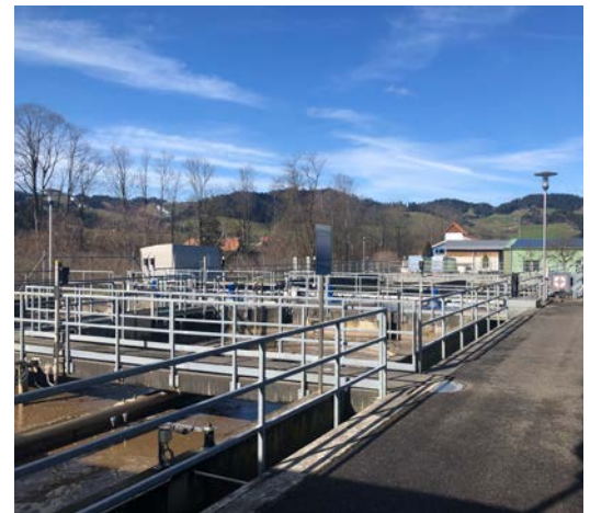
Figure 1: View over the nitrification of the plant
